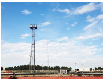
HIGH MAST LIGHT
